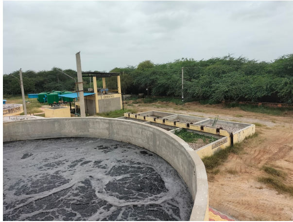
Photograph: Ventrovert, Sludge thickener and drying bed view near FAB Reactor, Wikimedia Commons, 2023. CC BY 4.0 ( creativecommons.org/licenses/by/4.0/ ); resized and recompressed. Sludge-path context, not a documented return-liquor event or company installation.
